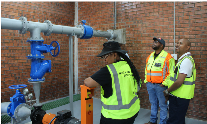
EXECUTIVE MAYOR ALDERWOMAN MP NKOSI, DIRECTOR CORPORATE SERVICES MR MS DLAMINI AND MUNICIPAL MANAGER MR M KUNENE DURING AN ONSIGHT INSPECTION OF THE BOOSTER PUMP STATION.
